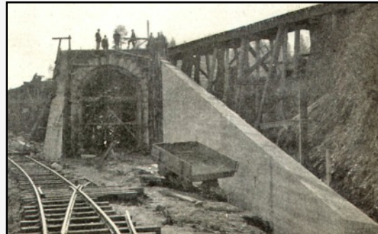
One of the tunnels added during double-tracking the Donner Route is the Applegate subway where the new Track 2 crosses under Track 1. See page 4 for more details. PSRHS collection
